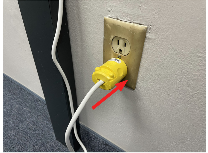
Power cable plugged into wall socket.
